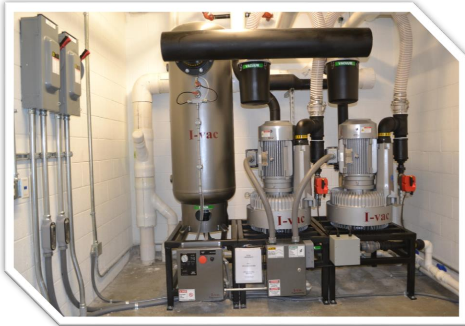
ABOVE: 60 Horsepower / 120 USER DUPLEX VACUUM SYSTEM
